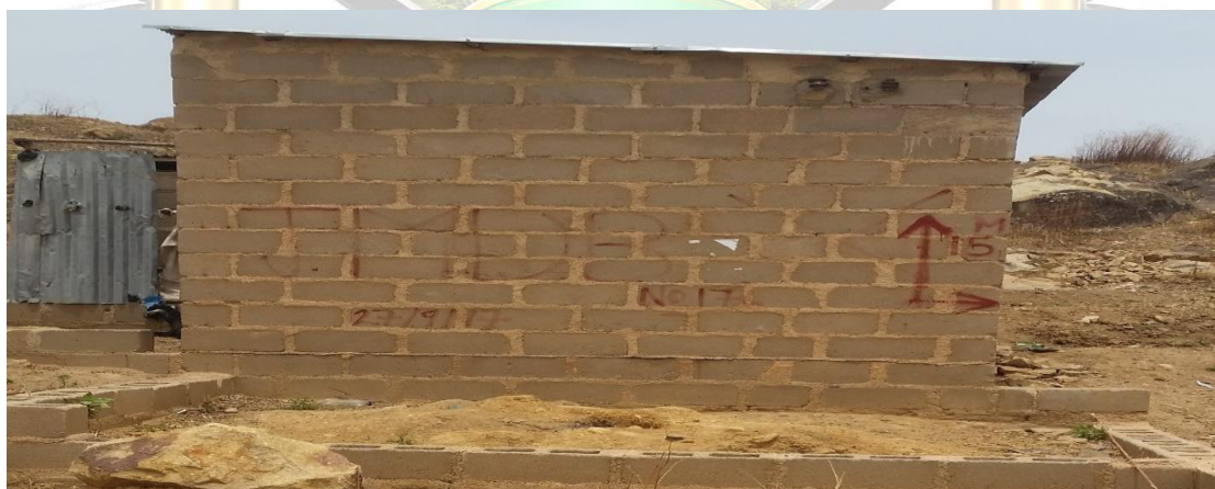
Figure 3a: Building Marked by Development Control Agency
