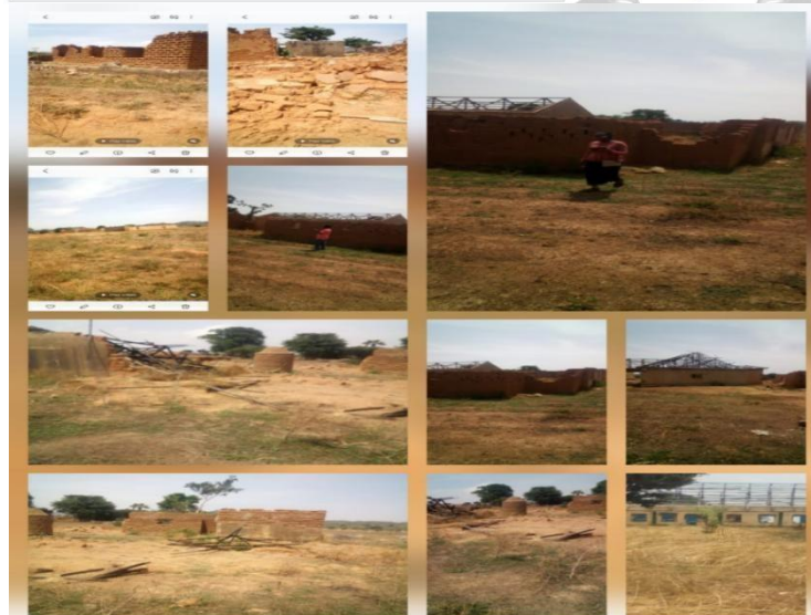
Figure 3: Type of Destruction Plate 1: Showing the extent of Houses Destroyed
